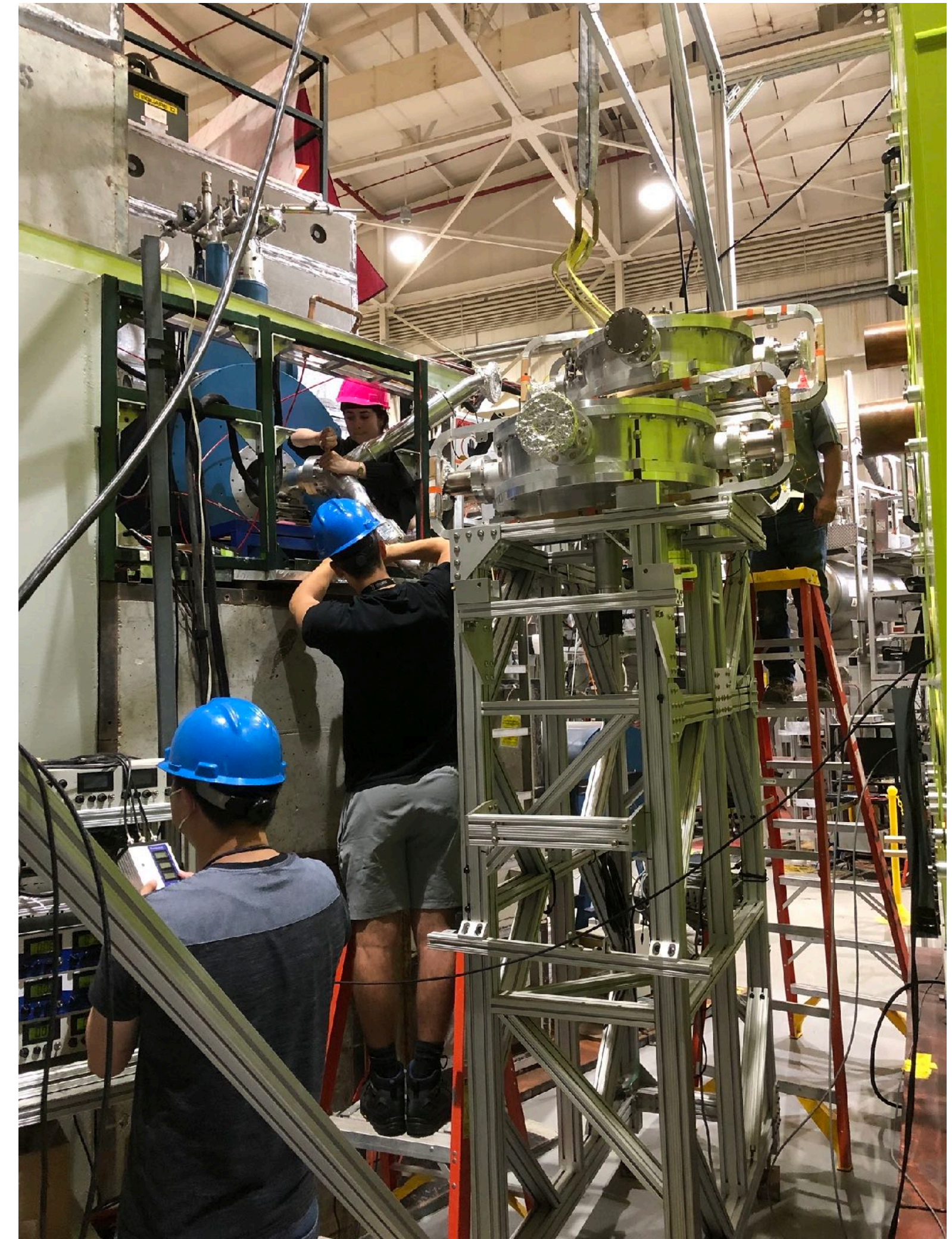
Switchers being installed
